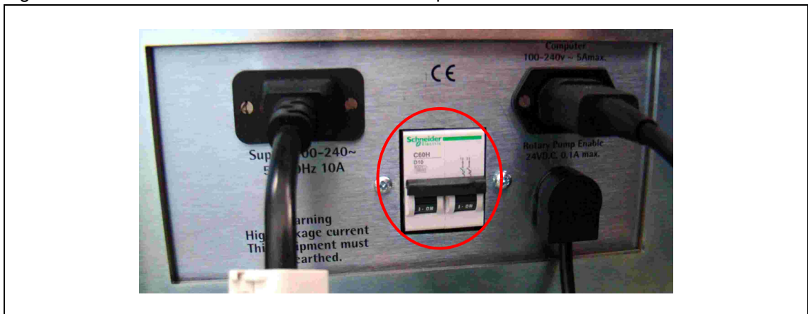
Figure 8.49 Circuit breakers shown in their closed position
